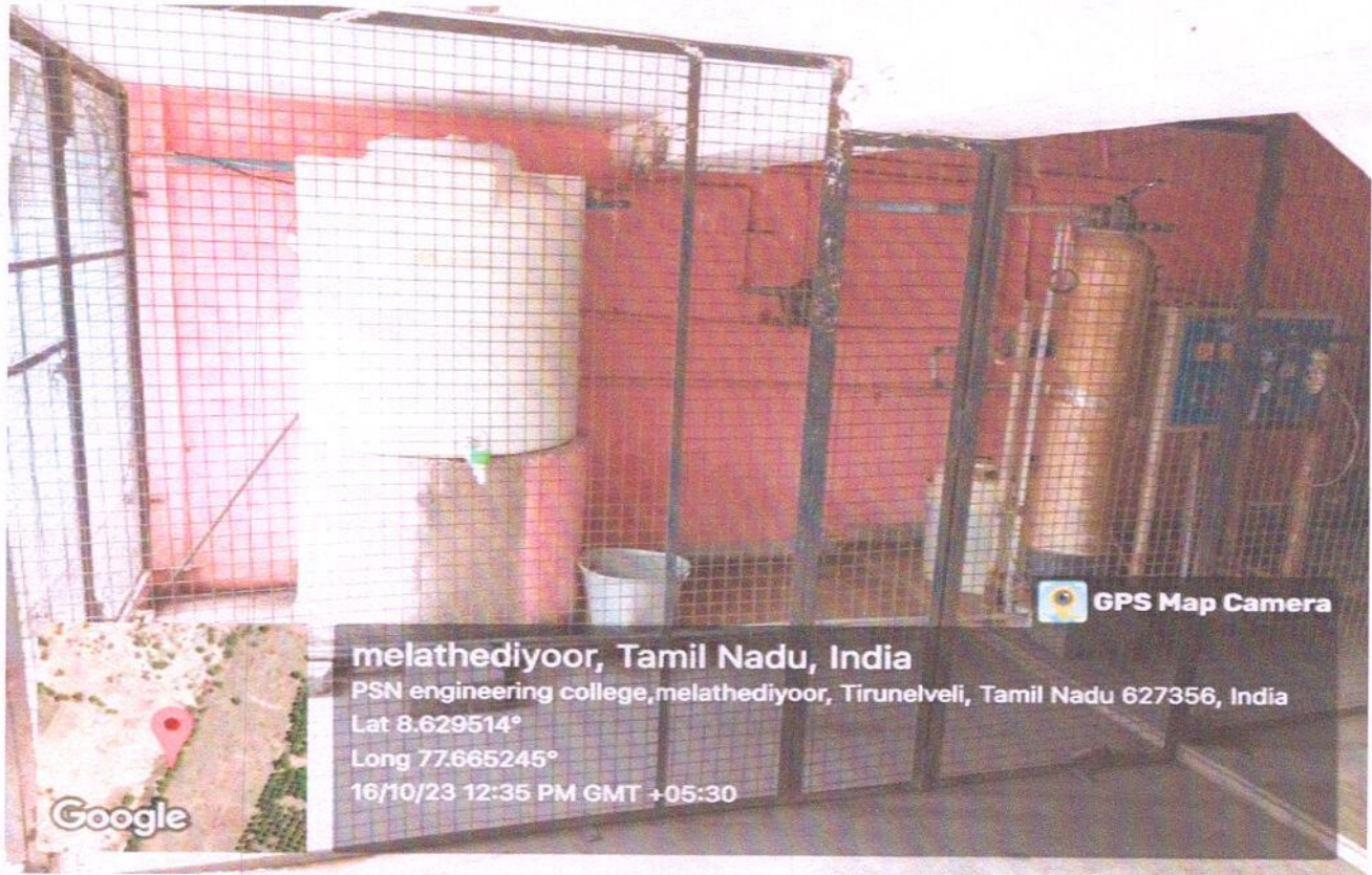
RO plant at PSNEC which is located at Main building ground floor
